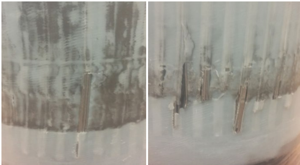
Figure 5-13 Cracked modulating ring
