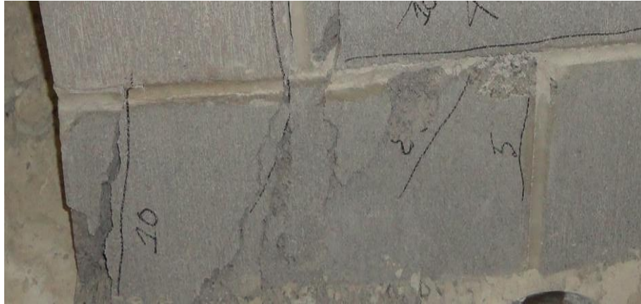
Figure 5.24 Cracking in the South Toe of Wall 7-B
